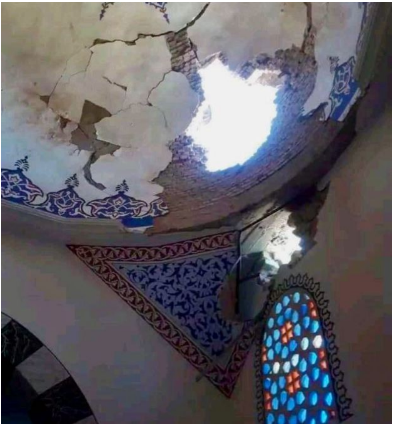
Negash mosque – one of the oldest in Ethiopia – damaged by shelling
